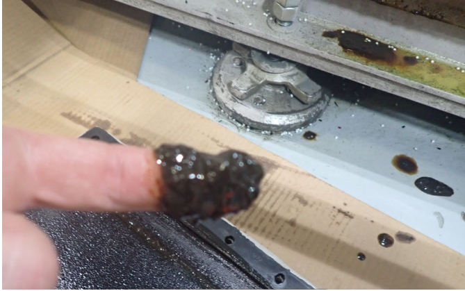
1 an inch of sludge in a hydraulic reservoir
