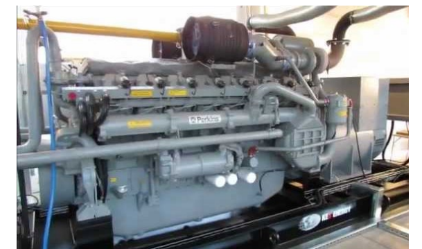
Photo still: (10) 1 MW Perkins 4016-61 TRS Natural Gas Genset- Kes Energy - YouTube
