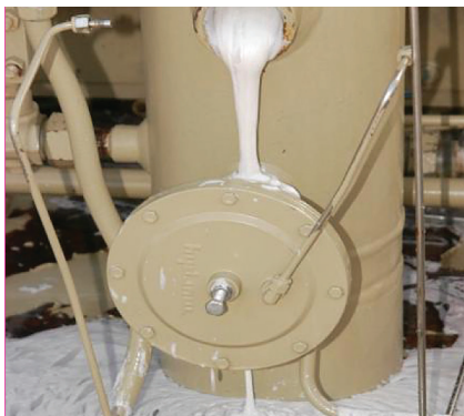
Emulsion in the scrubbers.
